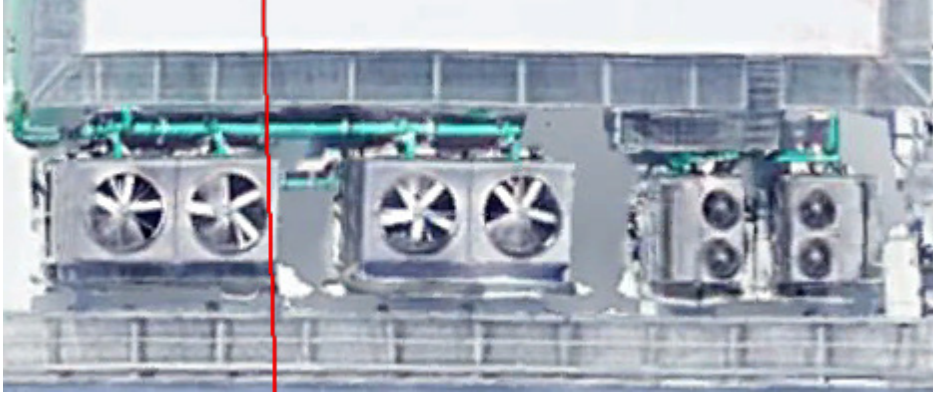
Figure 33: Cluster of CTs on a rooftop. This could be considered one CT cluster, three CT groups, or six independent CTs. Numbering schema should be consistent throughout your identification process.
