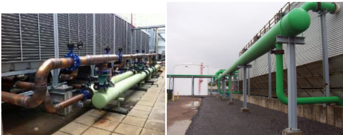
Figure 10: Colored water pipes.
