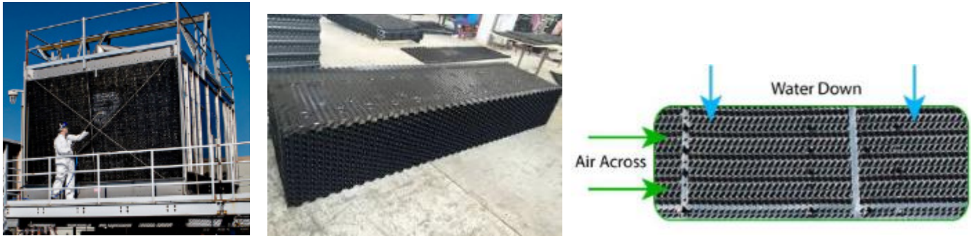
Figure 3: Examples of CT fill (Left: worker spraying fill on side of CT; Middle: fill removed from CT; Right: image of fill showing movement of water and air).
