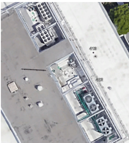
Figure 3: Two non-cooling towers with 10 fans per unit, and four CTs with one fan each (note the green water pipes serving the CTs).
