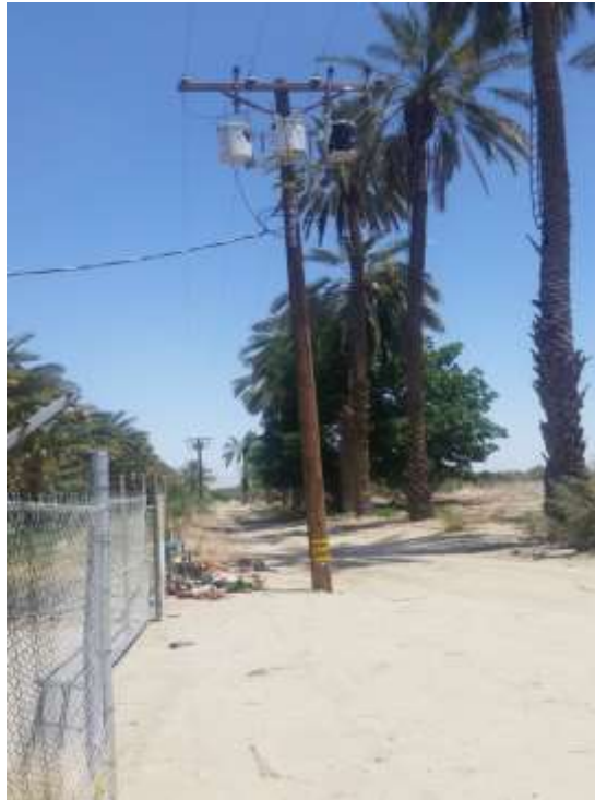
Exhibit 3. Location of truck (adjacent to power lines).
