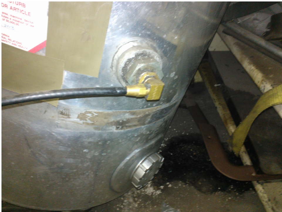
Exhibit 5. The air hose connected to the hydraulic tank.
