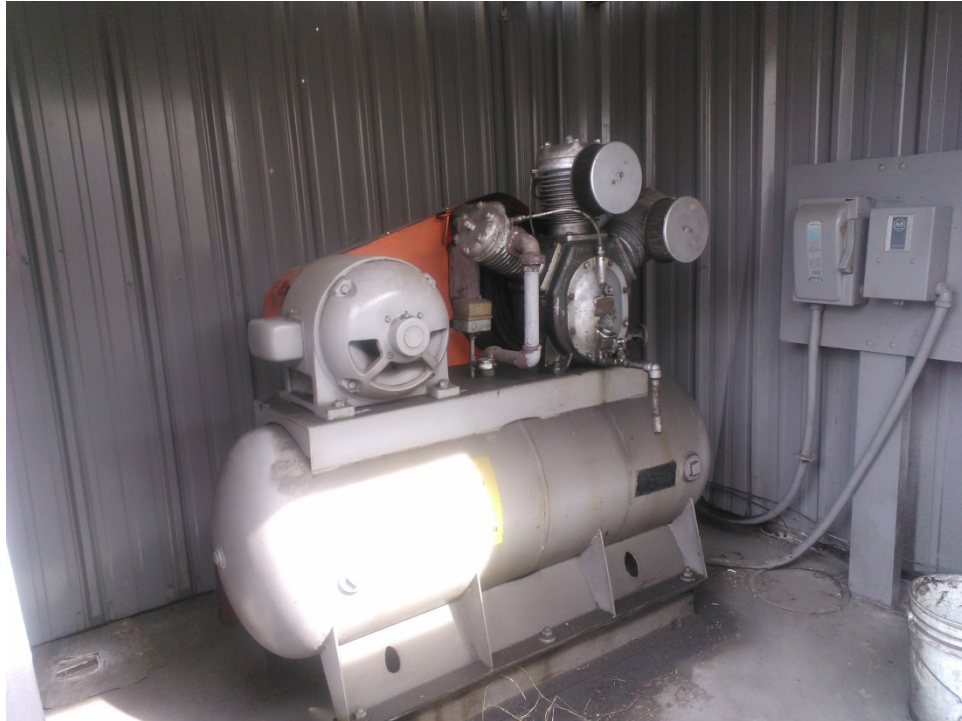
Exhibit 6. The air compressor that supplied air to the entire shop.
