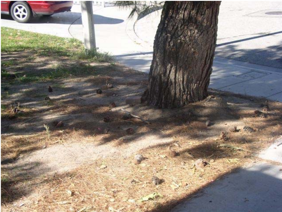
Exhibit 6. The ground at the base of the pine tree.
