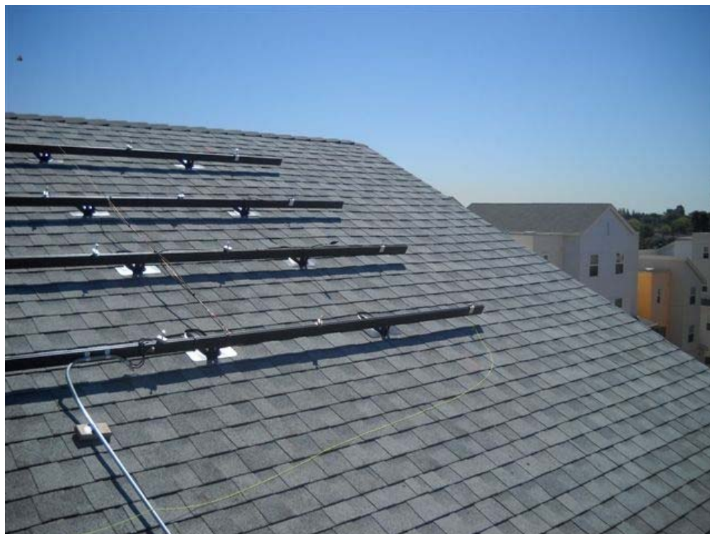
Exhibit 2. The mounting brackets for the solar panels and the roof's edge where the victim fell.
