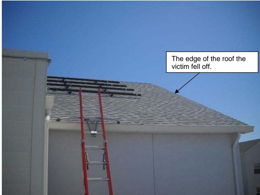
Exhibit 1. The roof edge the victim fell from.
