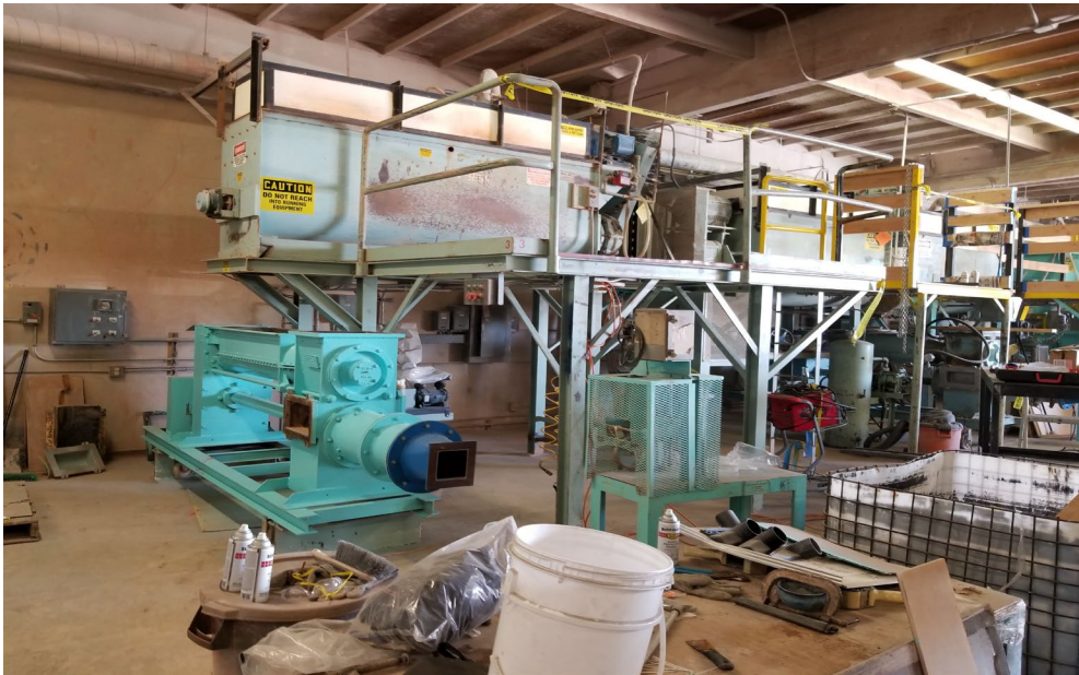
Exhibit 1. A pug mill identical to the one involved in the incident.
