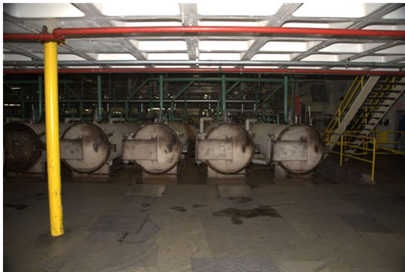
EXHIBIT 1. The pressure cooking and sterilization section of the processing plant.
