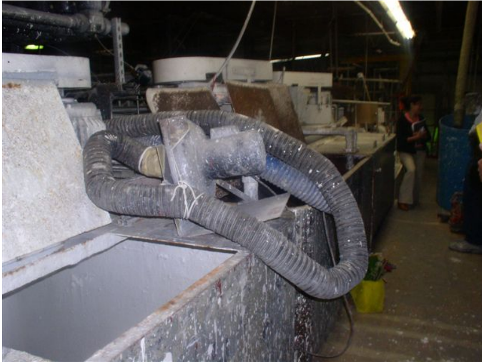
Exhibit 6 - The air pump and hoses that were used to remove contaminated air from the tank.
