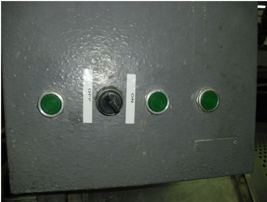
Exhibit 6. The buttons on the control panel.
