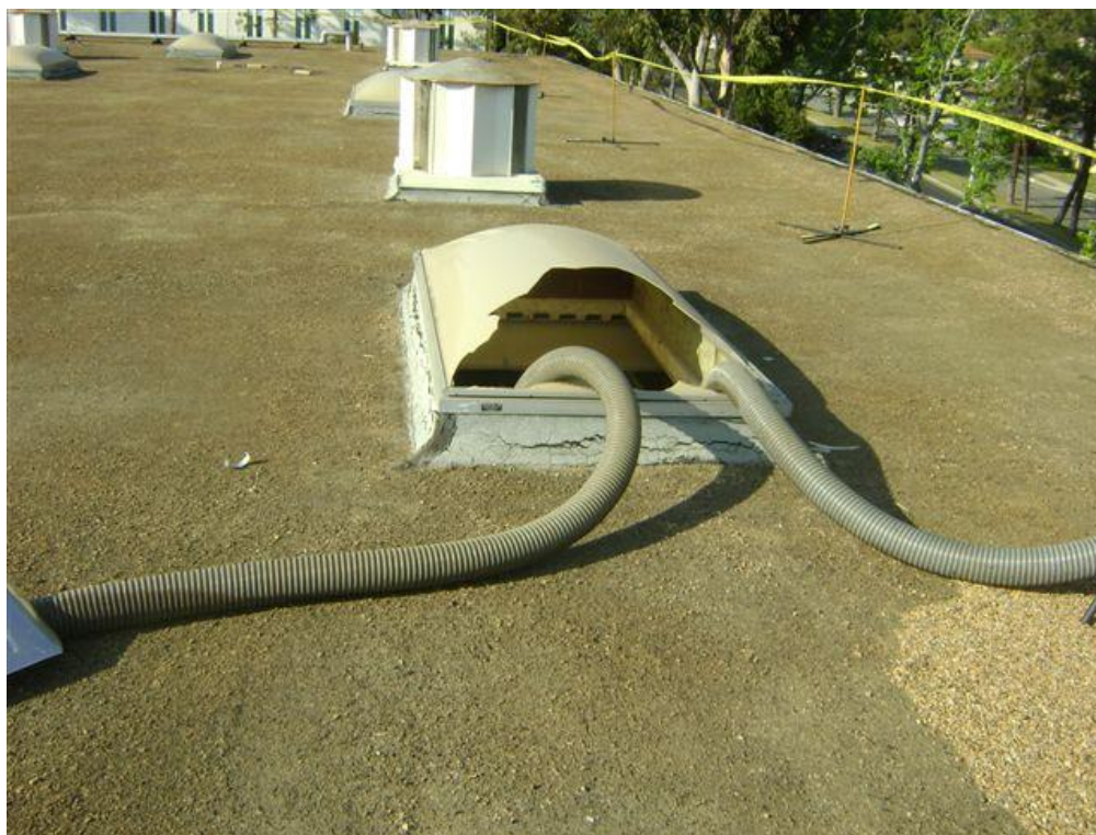
Exhibit 3. The skylight the victim fell through.
