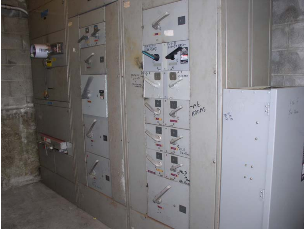
Exhibit 2. A picture of the electrical room where the panel was located.
