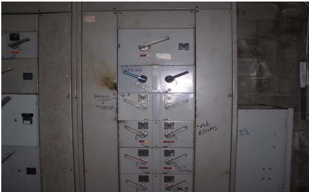
Exhibit 1. A picture of the electrical panel involved in the incident.
