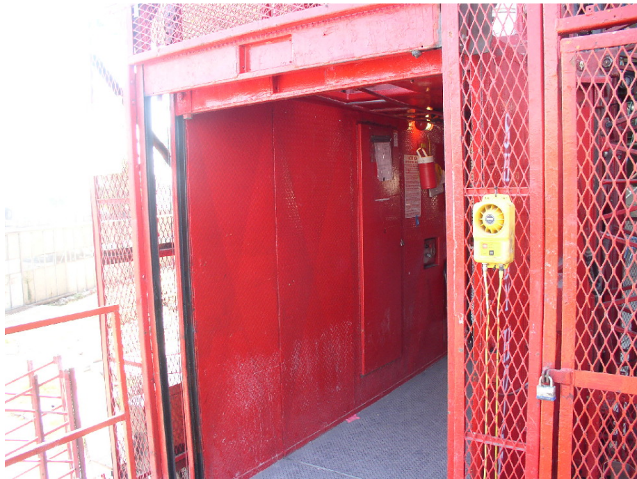
Exhibit 4. A picture of the elevator.
