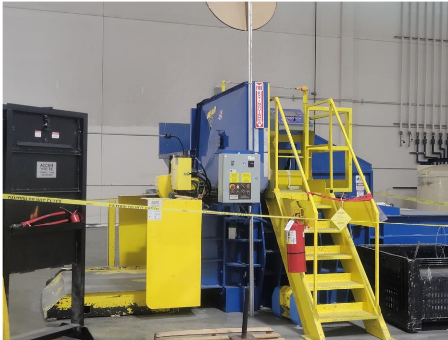
Exhibit 5. The stairs leading to the control panel. Photo by CA/FACE program.
