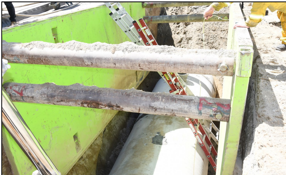
Exhibit 5. The ladder the victim was going to use to exit the trench. Photo courtesy of police department.
