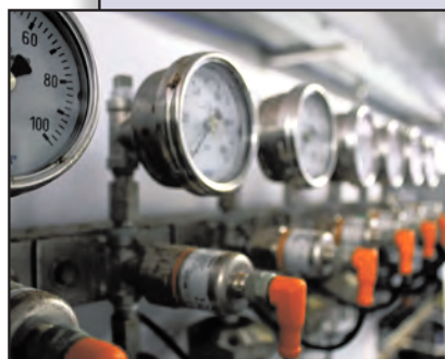
Pressure gauges at a waste water treatment plant
